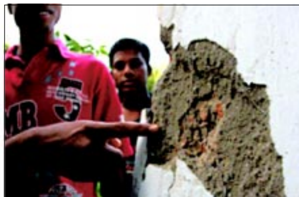
Figure 9.4: Residents examine a cracked wall of a building following last month's quake
