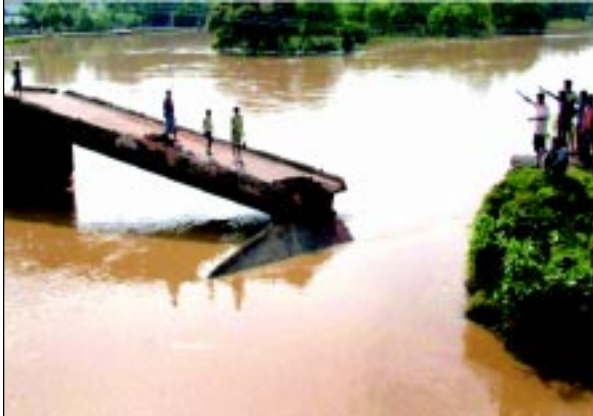
Figure 11.6: A bridge damaged in floods near Gudhikhal village of Balasore District in Orissa Photo source: Times of India
