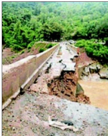
Figure 10.13: Collapse of strategic road bridge in Himachal Pradesh, India
